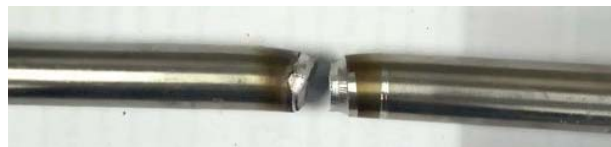
FIGURE 4. Fracture occurs exactly at the joint during the cross weld tensile test, represents real joint strength
