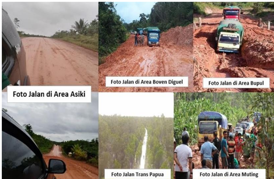
Figure 2. The condition of the roads is damaged in several areas of Boven Diguel Regency
