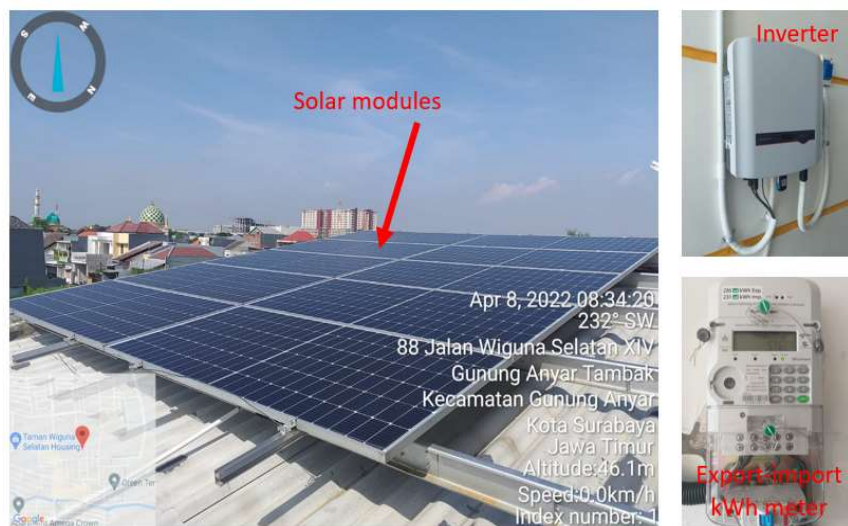
Figure 1. Photograph of PV system components
