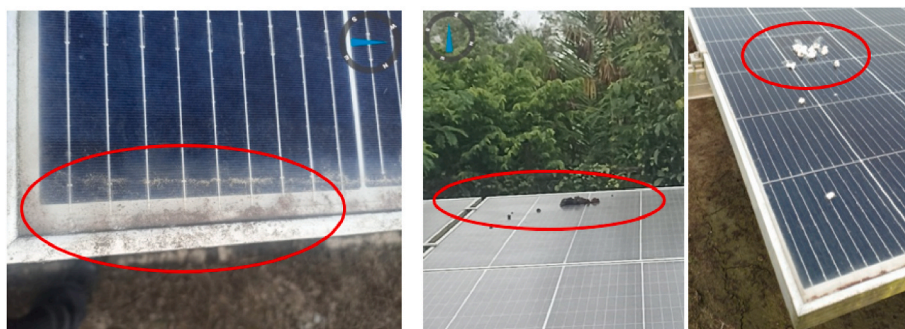
Fig. 5. Unexpected soil and dirt on the PV Module.
