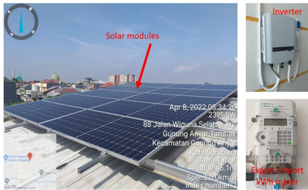
Figure 2. Photograph of installed PV System Components
